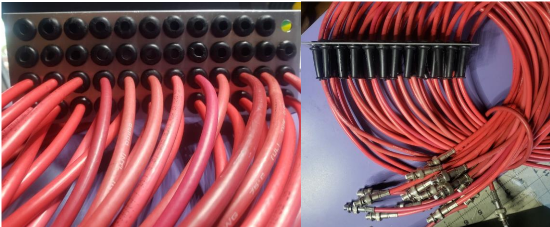
Front (left) and top (right) views of SHV cables pulled through adapter panel grommets
